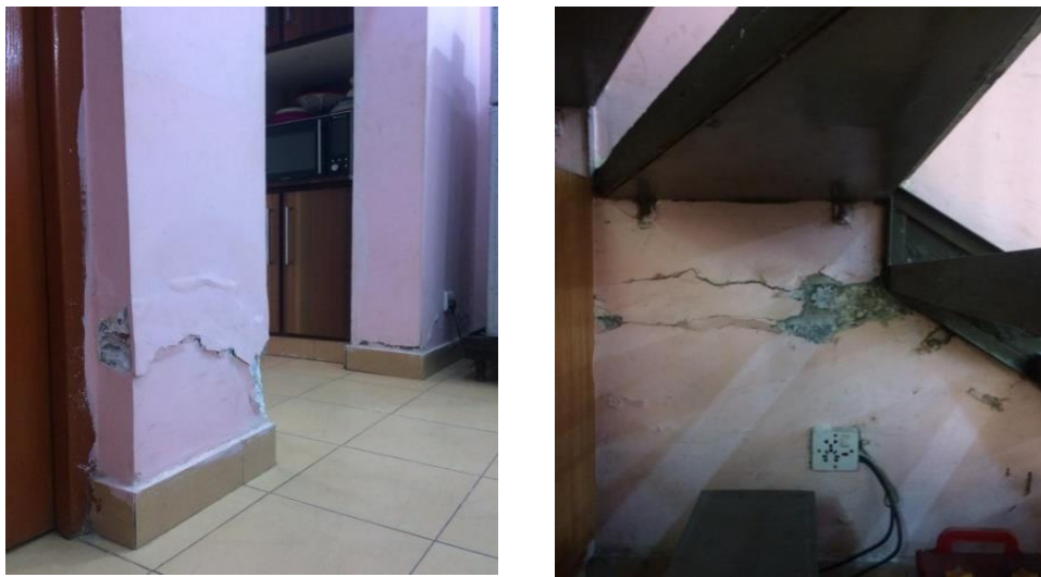
Figure 7: Cracks on the wall in one of the houses, Ashiana Housing Project, Lahore
