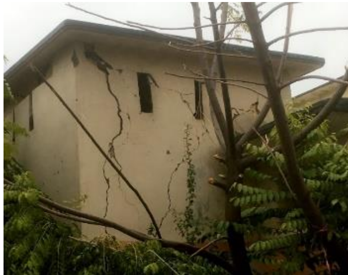
Fig 12: damage by the 2005 earthquake (Author, 2019)
