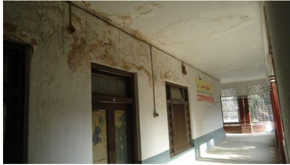
Fig 21: Leakage issues (Author, 2019)
