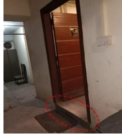
Figure 5 Step at door
